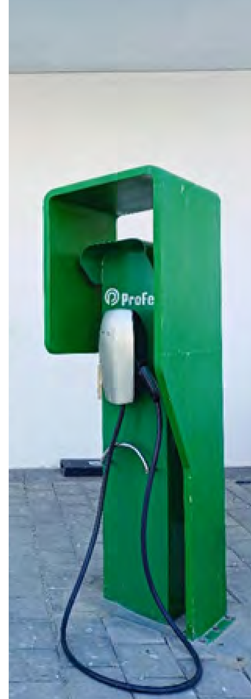
EV Charger Meydan
